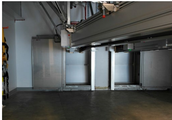
Figure 6. Fire Doors in NFN Tunnel Area
