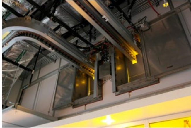
Figure 5. Fire Doors in NFX Link Area
