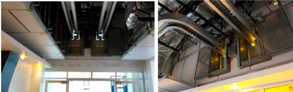
Figures 10 & 11. NFX Link Fire Door Set- Ceiling Tiles Removed
