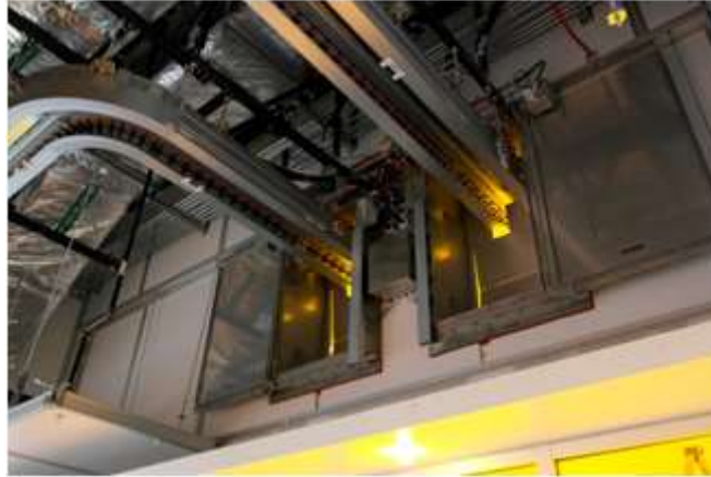
Figure 5. Fire Doors in NFX Link Area
