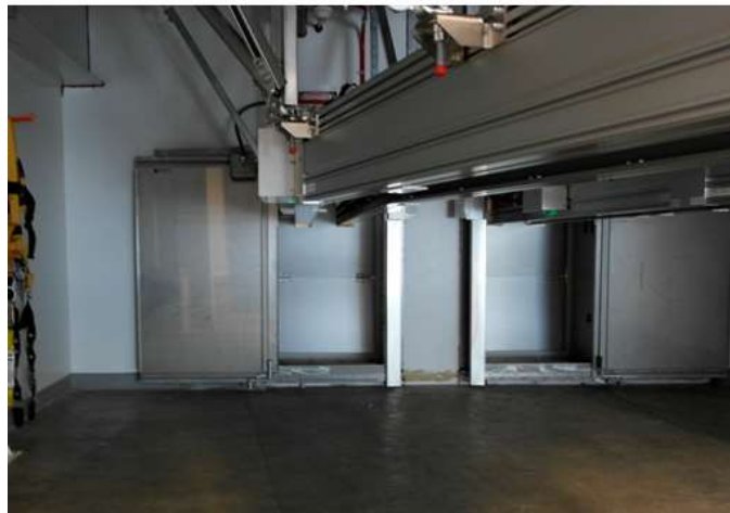
Figure 6. Fire Doors in NFN Tunnel Area
