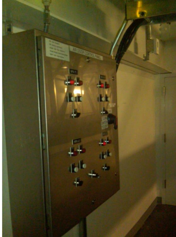
Figure 2. Air Door Controller
