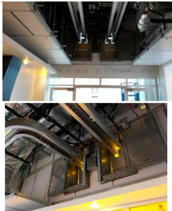
Figures 10 & 11. NFX Link Fire Door Set- Ceiling Tiles Removed
