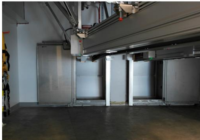
Figure 6. Fire Doors in NFN Tunnel Area
